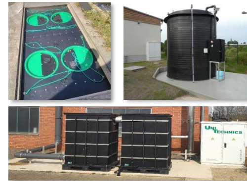
Dosing & Exhaust Air Treatment
