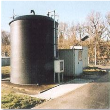
Chemical Dosing Station (Fe 2+ )
