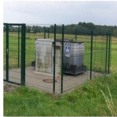
Chemical Dosing Equipment (NO 3 - )
