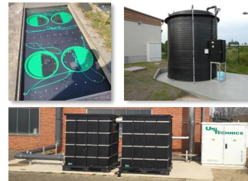
Dosing & Exhaust Air Treatment
